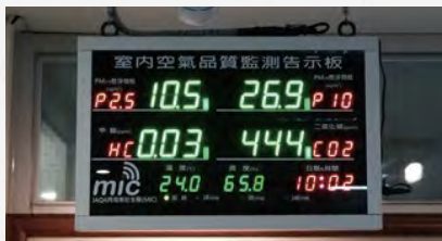
▲ Indoor air quality real-time monitoring panel
