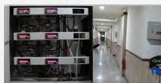
▲ 1st Student Dorm & General Dorm installed with 266 digital meters
