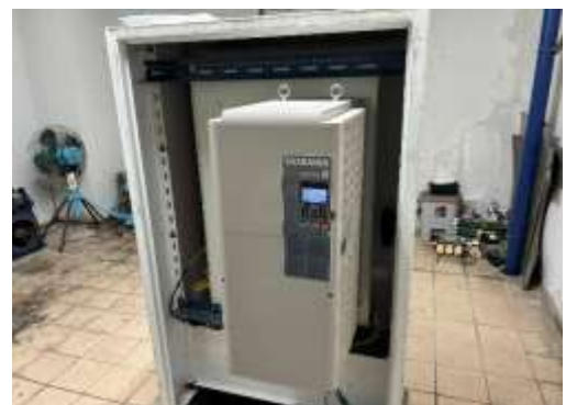
Energy feedback system of the elevators of the Student's 1 st Dormitory
