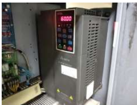
Energy feedback system of the College of Law's elevators
