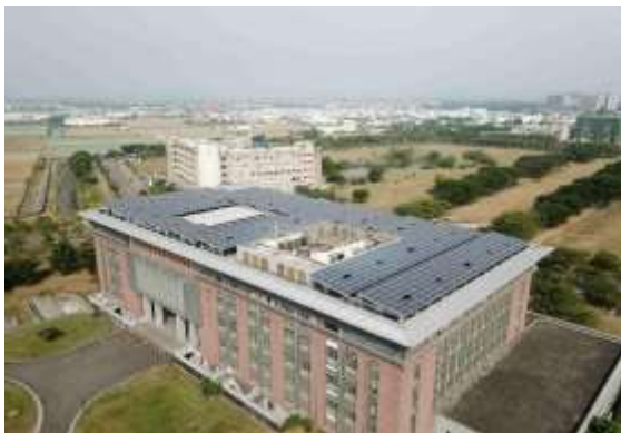
Solar PV system
